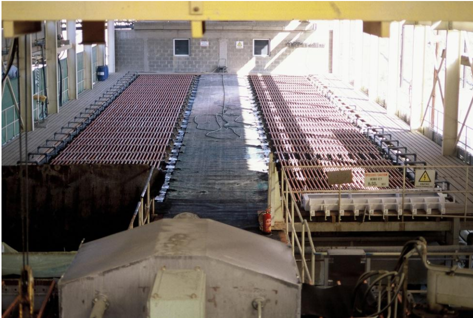
Electrowinning plant- tank house
